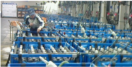
Charging process of storage batteries
